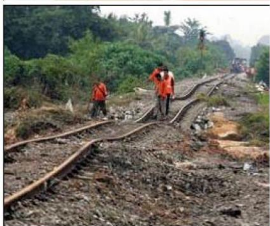
JOHOR: Railmen checking out the damage caused by the floods in Segamat. NST Pix
