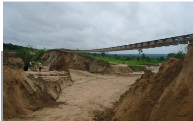
Severe damage to bridge (missing middle support)
