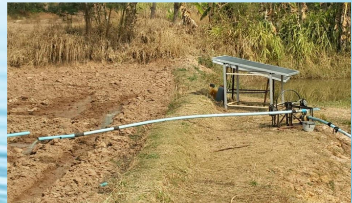
Solar cell water pump
