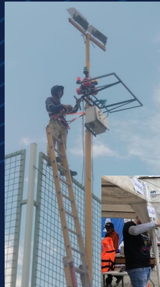
The Duran Early Warning System (SAT) was ready in April 2023
